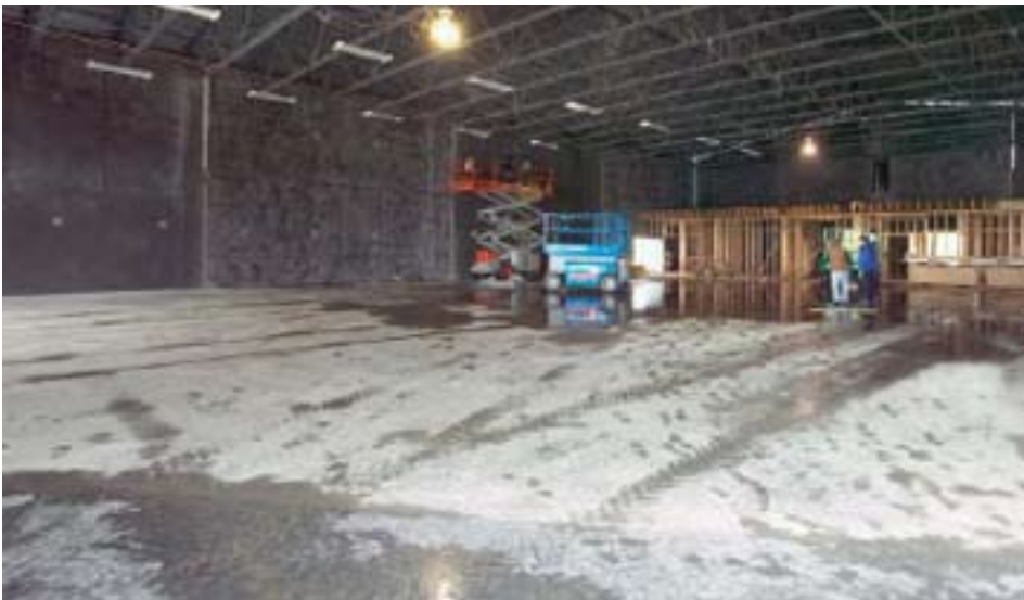
Pictured above during construction, the Parr Lumber floor features no joints, thus no curling to create hazards and wear on the forklifts that carry loads over it.
